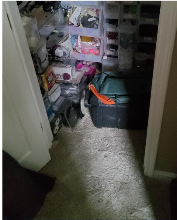
Cityworks WO-23007929 – Photo of damaged carpet at a home. (Image:16751163193896973529692903738232.jpg)
