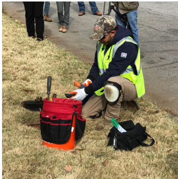
DeKalb is on track to replace 30,000 water meters during the first year of the New Day Water Meter Exchange and Upgrade Initiative.
