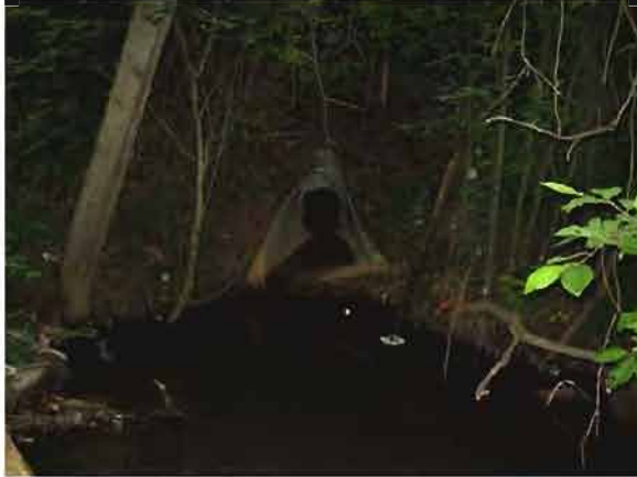
Site 63. CMP discharging to stream.
