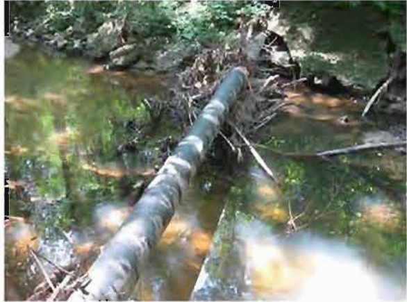
Site 201. Log jam at a pipe crossing.
