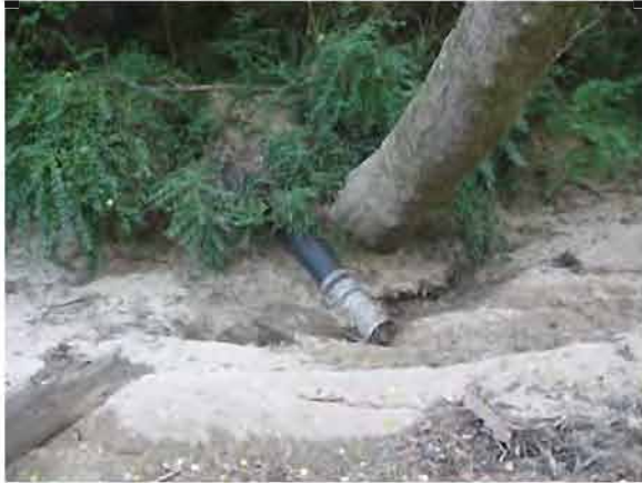
Site 125. Section of French drain.
